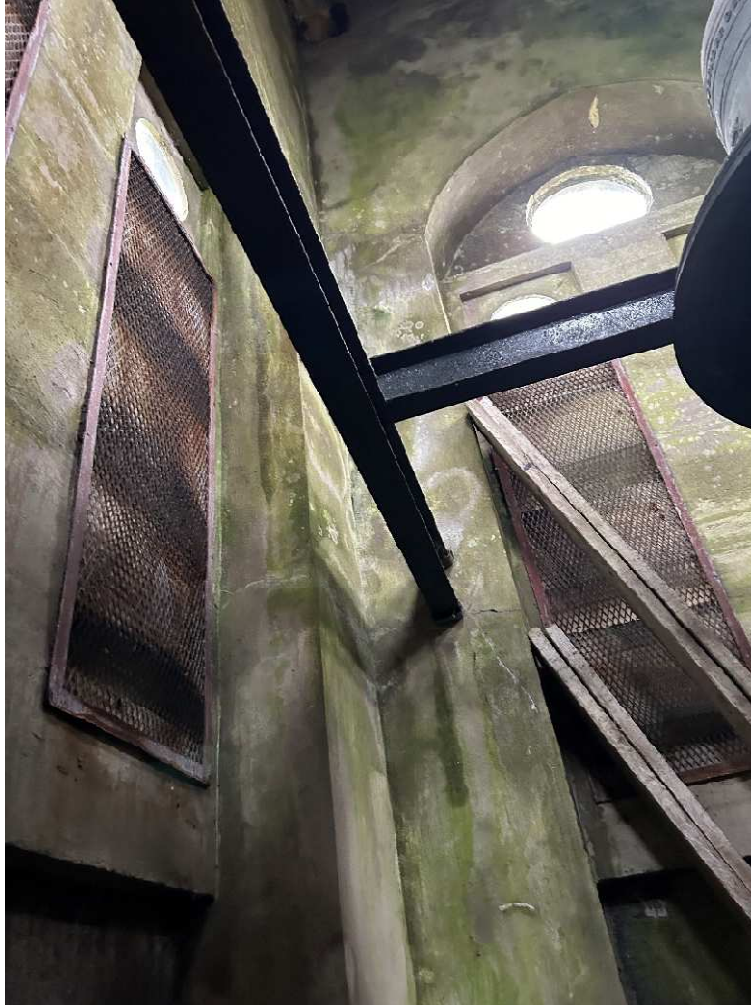
Photograph 003 Showing internal photograph of the Bell Tower at the bell level, water ingress on wall walls noticed on the internal plaster.
