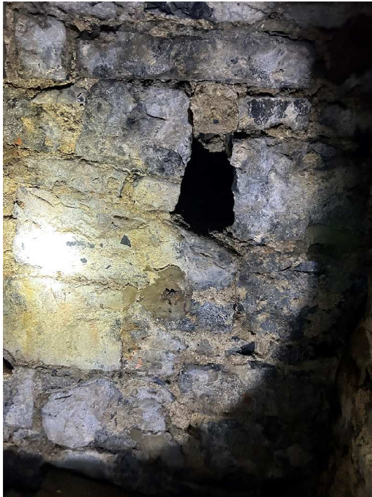
Photograph 004 Showing internal photograph of the Bell Tower lower level at exposed random rubble stone walls, all face of the exposed stone are wet & some having dripping water for surface water.
