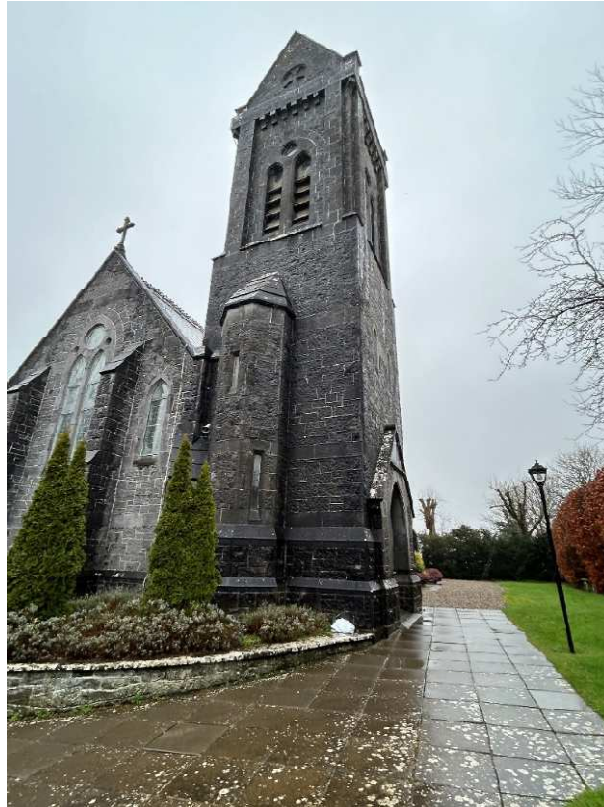
Photograph 001 Showing the external saturated Bell Tower.
